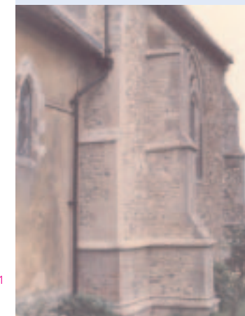
A new quoin (the outer corner of a wall) inserted at Tilty Church, Essex. The use of new stone, costly and also involving loss of historic fabric, was necessary after the gutter, hopperhead and rainwater pipe had become blocked and remained so for several years encouraging plant growth and decay in the wall.
