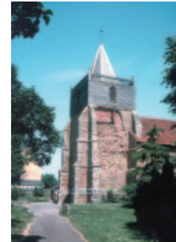
A blocked hopperhead and rainwater pipe caused water to run down the wall of the tower at Great Clacton Church, Essex. After a number of years this water led to the collapse of areas of the face (of Septaria stone). Rebuilding involved scaffolding the whole of the south face of the tower at a cost of many thousands of pounds.
